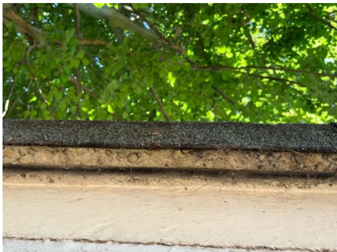
Figure 20: Concrete roof offers no bat access
