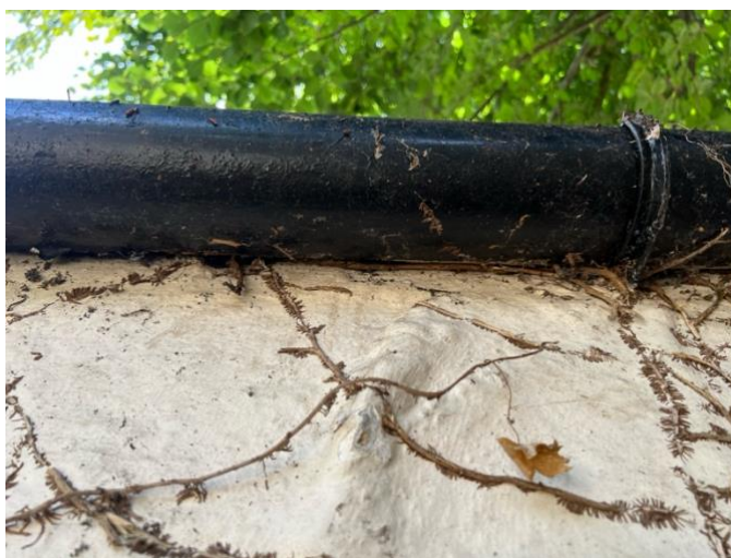
Figure 23: Guttering flush to the wall face
