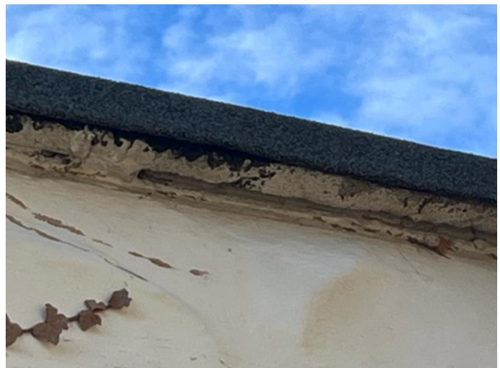
Figure 27: No gaps under overhanging roof felt
