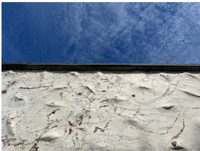
Figure 21: No gaps into wall top or under roof felt
